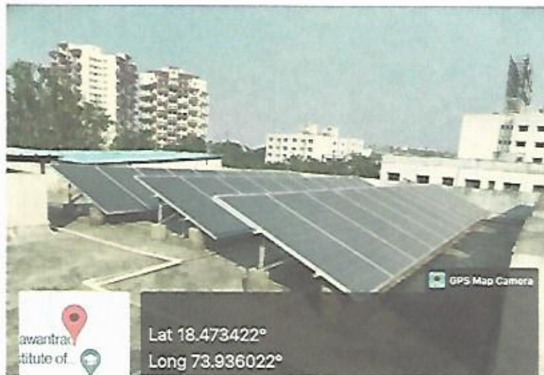
Photograph of 3 kWp Roof Top Solar PV Plant:
